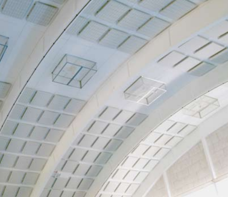
STARK Sport absorbent mounted in the ceiling in a sports centre.
